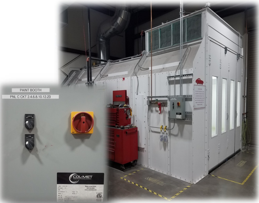
The COL-MET Auto Refinishing Booth installed in the New Addition of 6 years ago.
